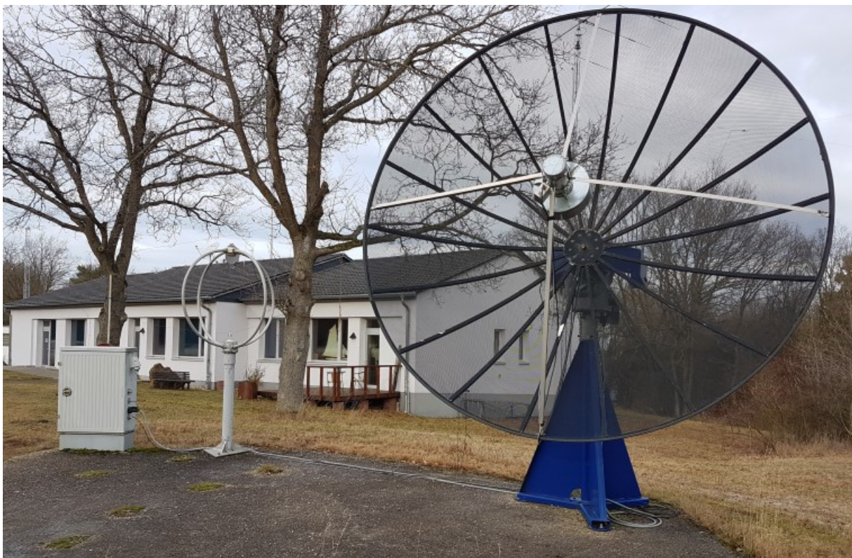
Figure 2: The dish and the outdoor cabinet. The loop antenna in between is used for other purposes and is not part of this installation
